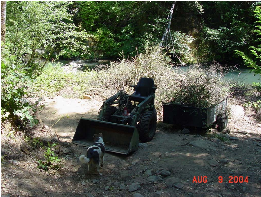
Photo courtesy USFS: use of heavy equipment to clear brush and move dirt, which is not allowed under suction dredge permit regulations
